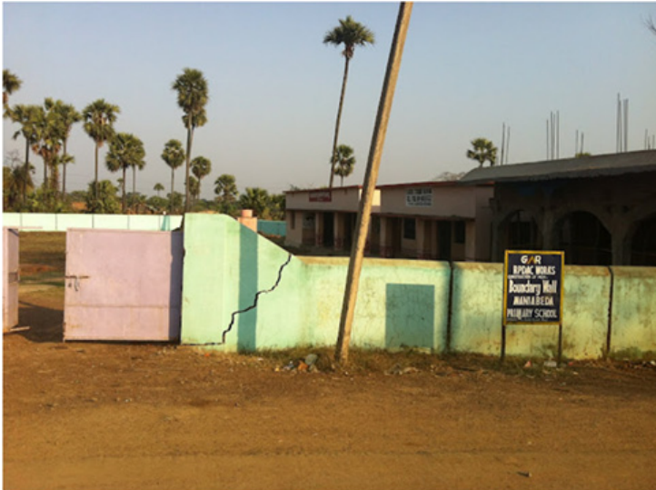
The school boundary wall constructed by GMR under its CSR. It shows the quality of the work. The boundary wall has already developed dangerous cracks.
